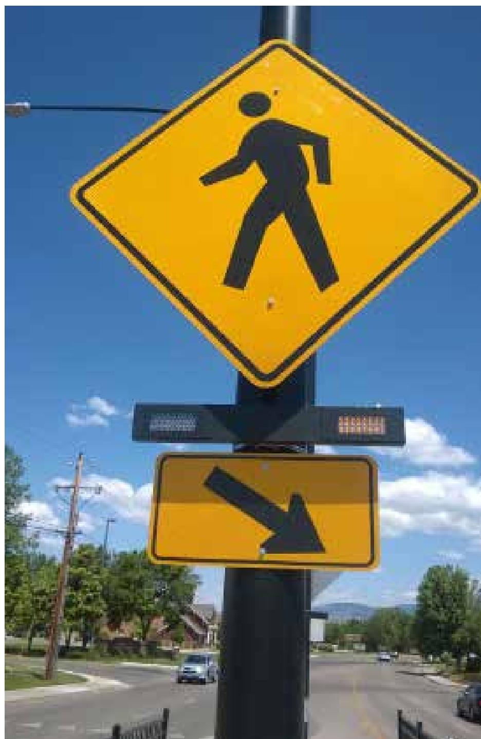
rectangular rapid flashing beacon
