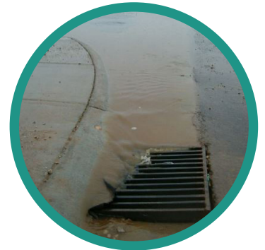
Construction Site Sediment Discharge
