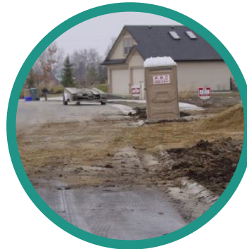
Poor Construction Site Practices
