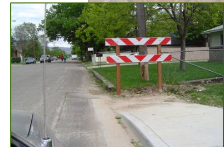
Missing sections discourage pedestrian travel and/or force pedestrians into street
