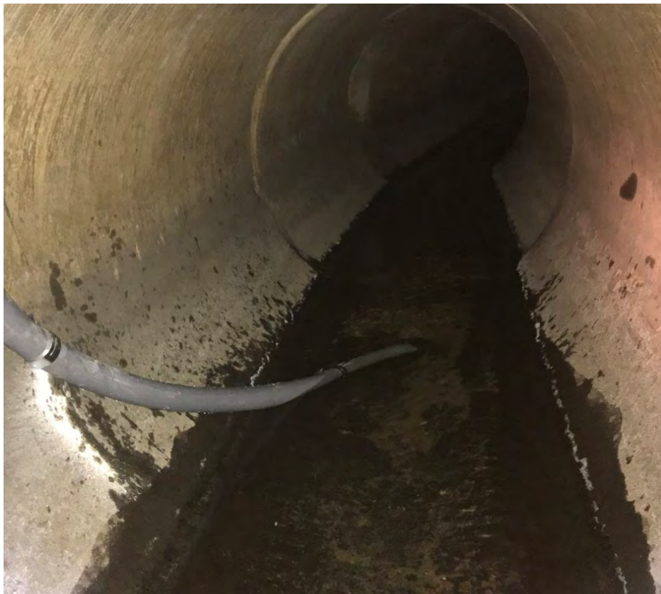
Figure 3-1. 16th and Front monitoring site installation
