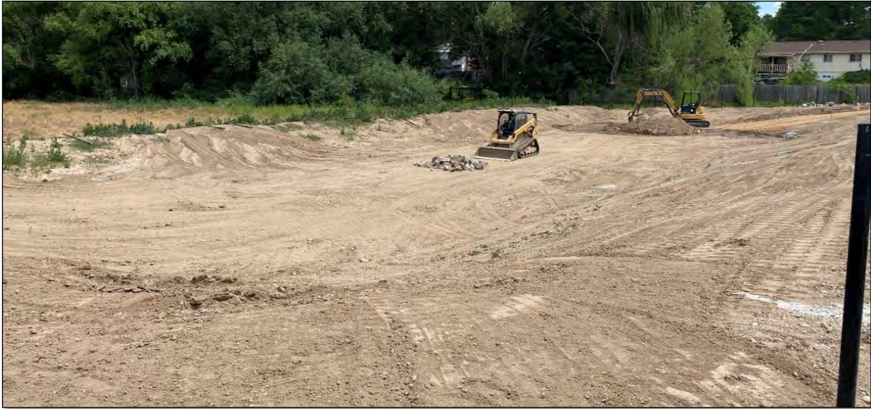
Photo 3: June 2023 – Photo taken facing northwest showing basin being prepared for installation of microtopography, topsoil, and concrete apron for the basin inlet.
