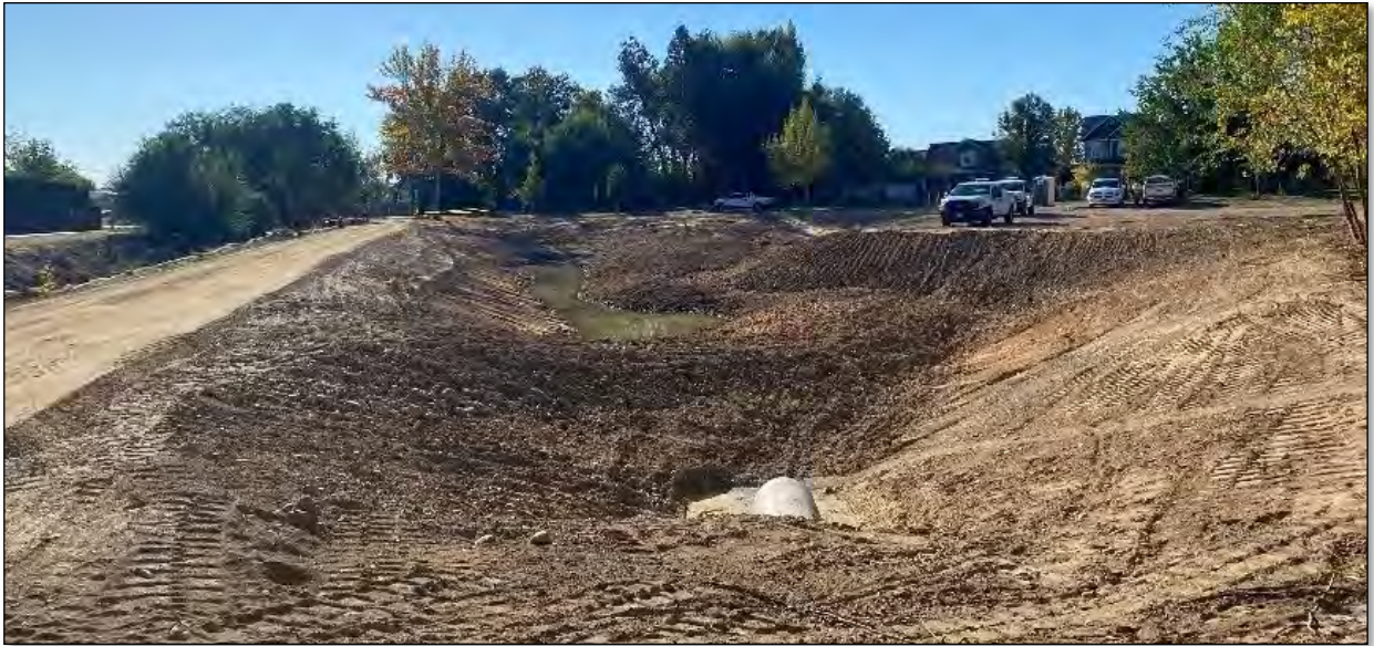
Figure 2: 10/09/2023 - Photo is taken facing south showing the rough grading and microtopography has been completed. The incomplete inlet pipe into the basin is shown in bottom of photo.
