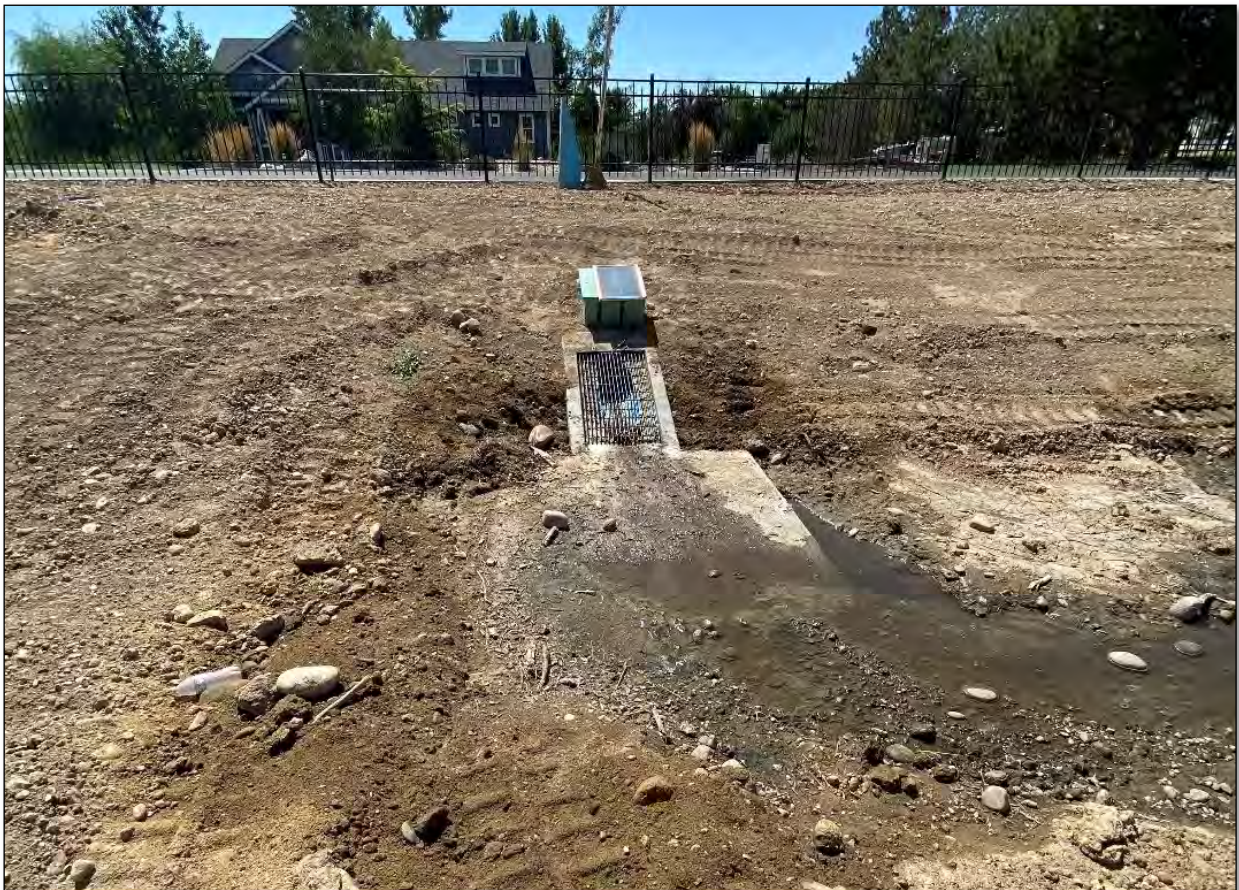
Photo 6: August 2023 – Photo taken from inside the basin facing south showing the completed inlet and installation of monitoring equipment. Note: Monitoring equipment was uninstalled in November 2023, due to water levels surcharging the inlet pipe.
