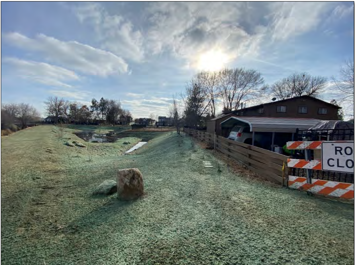
Photo 7: 12/19/2023 – Photo taken facing south showing containerized plants, hydroseeding, wood mulch and fence completed.
