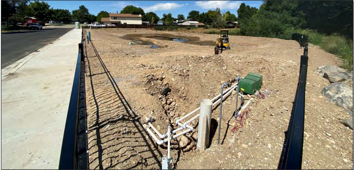
Photo 5: August 2023 – Photo taken facing northwest showing basin inlet, spillway, and fence installation complete and rough grading and irrigation system nearly complete.
