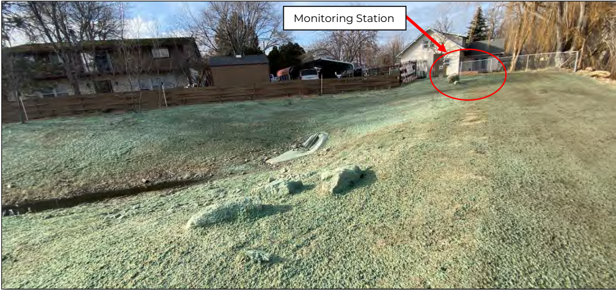
Photo 8: 12/19/2023 – Photo taken facing northwest shows the location of the monitoring station and the completed basin inlet.
