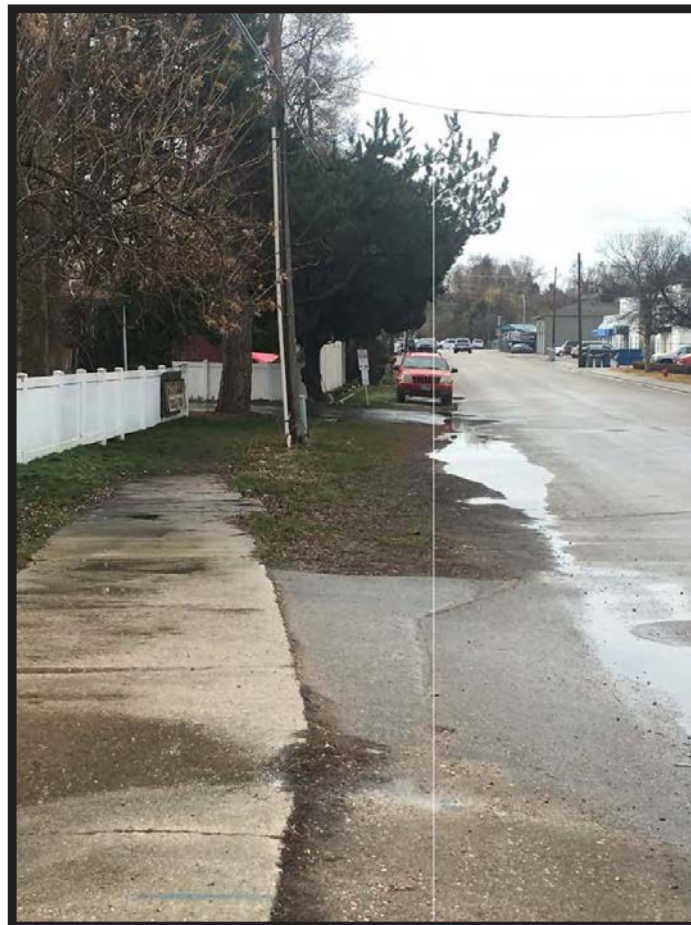
Picture 8 Sidewalk Missing on 38th Street
